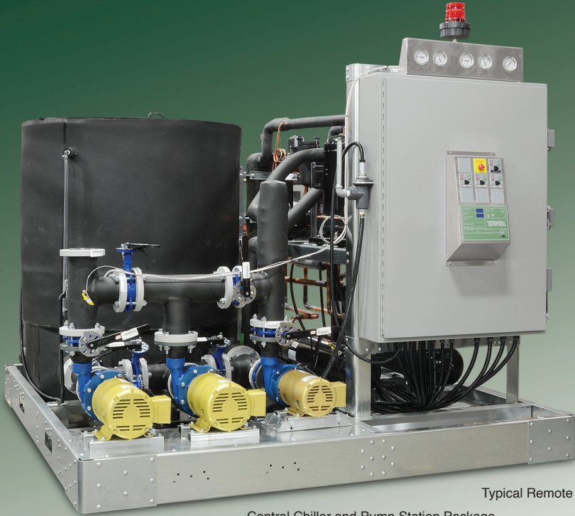
Central Chiller and Pump Station Package
